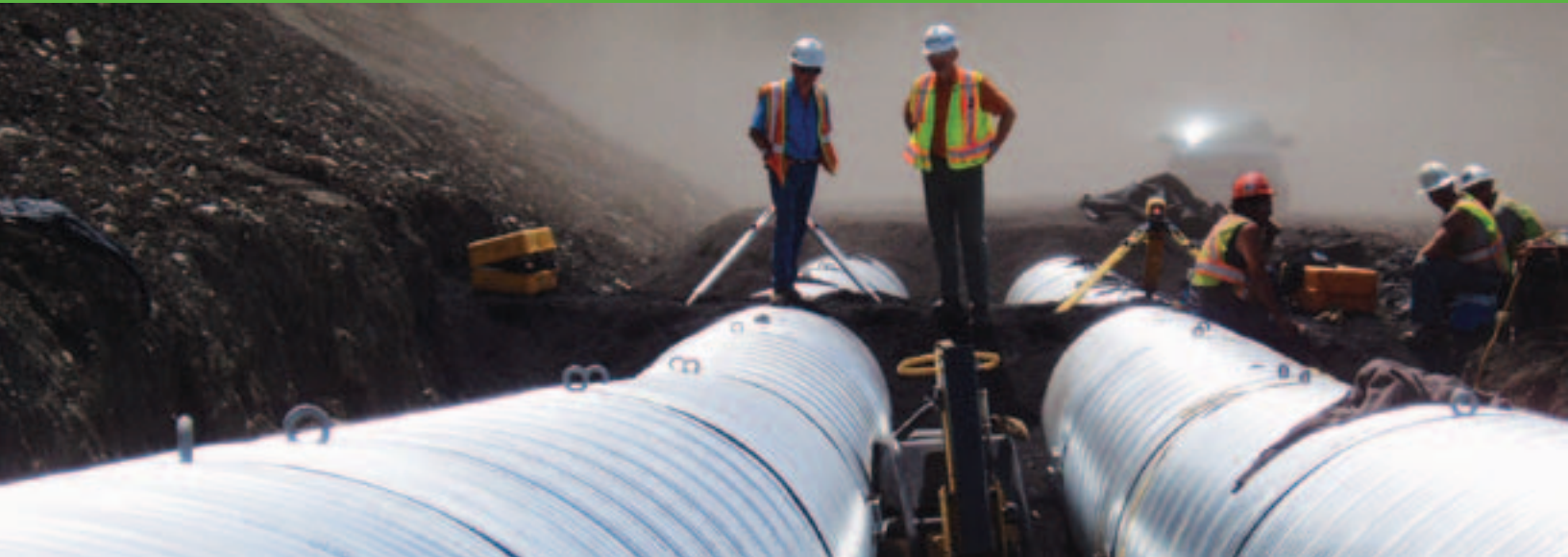
A water diversion under construction at one of our steelmaking coal operations located in the Elk Valley of British Columbia.
