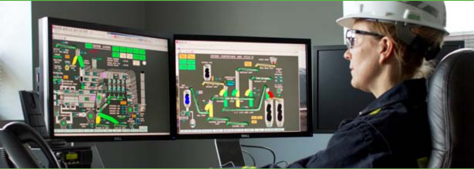
The dryer fan control room at one of our steelmaking coal operations located in the Elk Valley of British Columbia.
